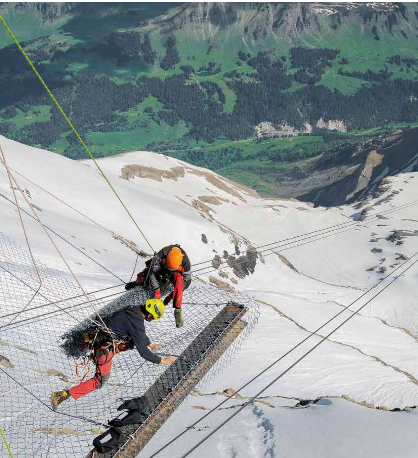
Installation of anchor points and safety nets for the reconstruction of the famous "La Botta" restaurant at Glacier 3000. Instalación de anclajes y redes para la reconstrucción del famoso restaurante «La Botta» en Glacier 3000. Les Diablerets, Switzerland (courtesy of Corde-Access SA, riggers Andrea Giuzzi & Julien Guisolan, ph. Ari Cretton).
